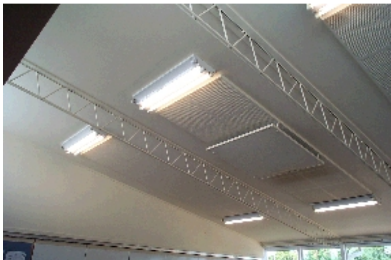
Figure 2: One of the classrooms after delamping. In each section, 6 fluorescent tubes were replaced with 3 triphosphor tubes. (Note: These rooms have excellent natural lighting and are never used at night.)
