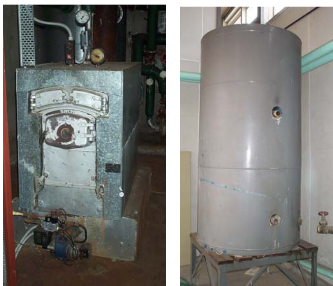
Figure 1: The old hot water boiler and hydronic storage tank that were disconnected. Energy wasted from these units came to 27% of total gas consumption. This is enough to supply gas to 12 homes in Melbourne.
