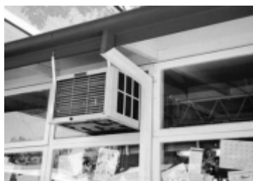
Window mounted air conditioning
