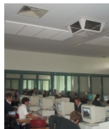
Evaporative cooling can be used in computer rooms
