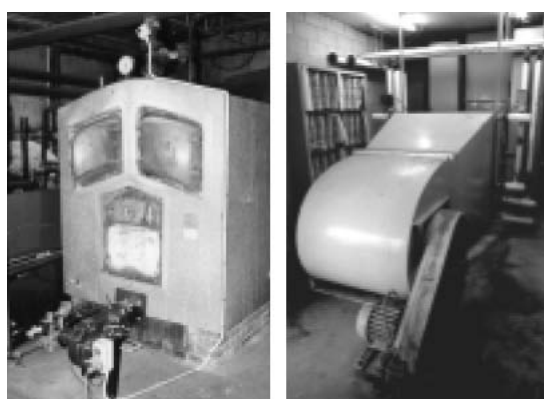
Typical boiler and fan coil unit common in schools
