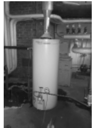
Centralised domestic hot water system
