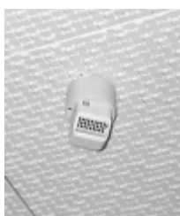
An ultra-sonic occupancy sensor
